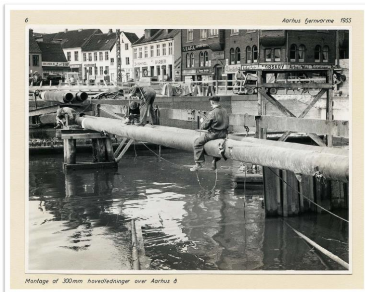
Figure 4: Deployment of 300 mm main pipes across the water in Aarhus, 1955. Source: Affaldvarme Aarhus; this was printed with permission.
